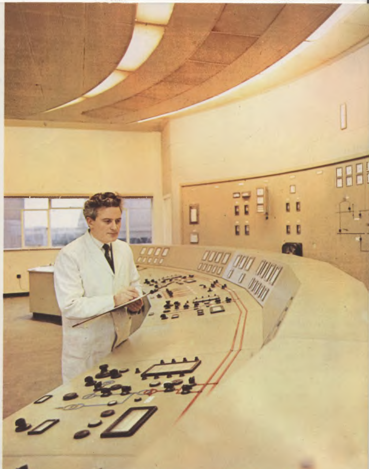
Electrical Control Room
